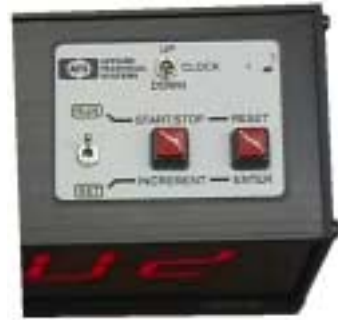
Set time switch panel
